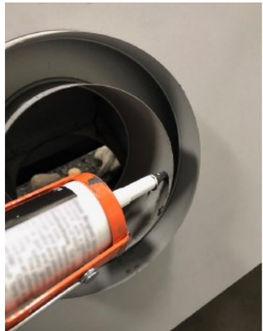
Figure 6.10 - Silicone Inner Exhaust on Fireplace
