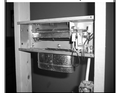
Figure 12.4, Installed Fan Assembly
